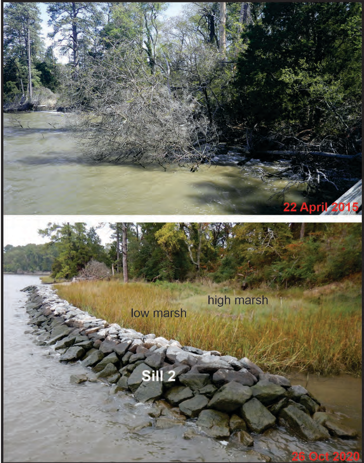
Figure 7-11. Pre-project shoreline showing an eroding bank with fallen trees (top); and Sill 2 about 4.5 years after construction showing a lush marsh (bottom). Photo credit: Shoreline Studies Program, VIMS.
