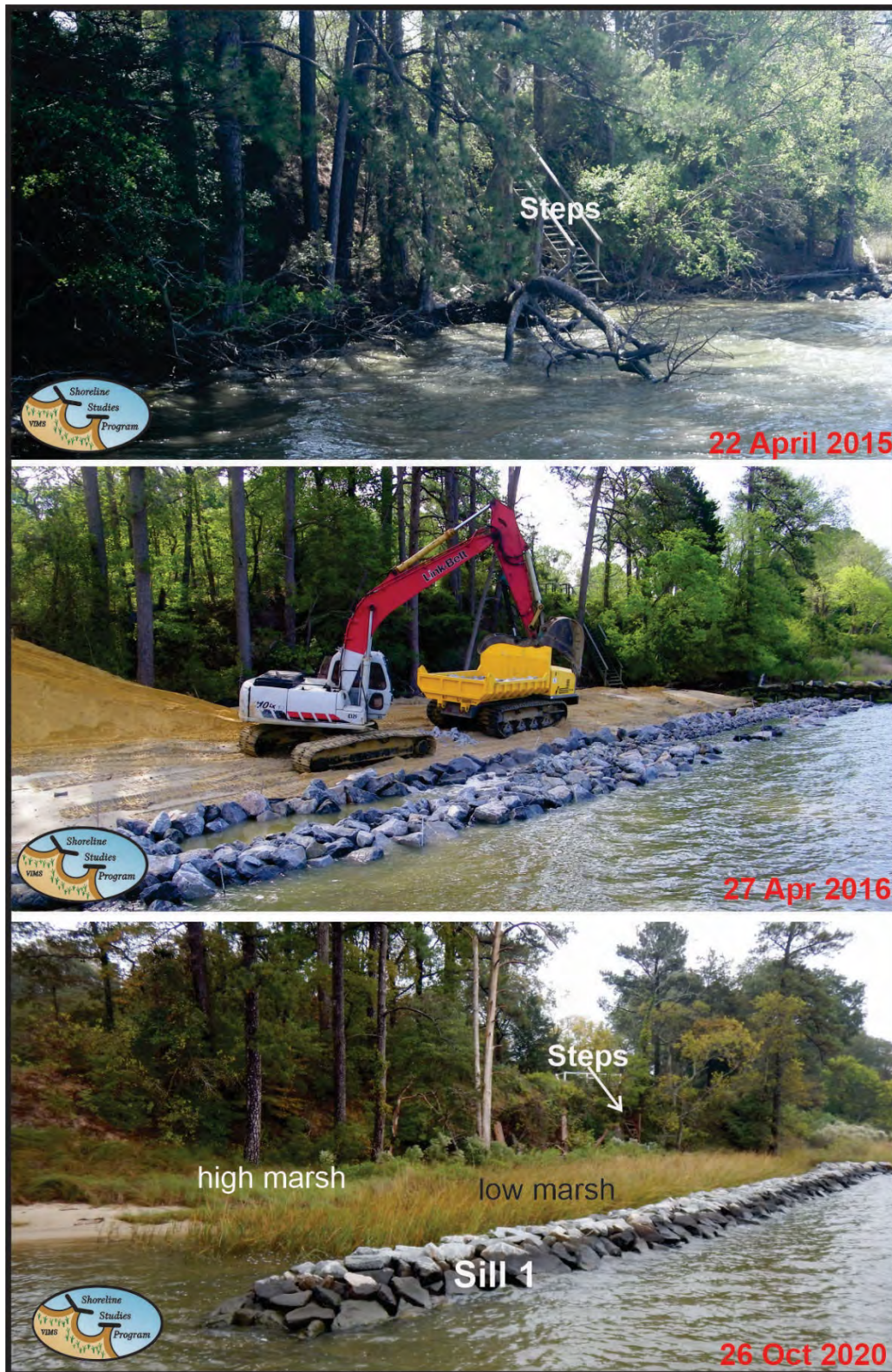
Figure 7-12. Pre-project shoreline showing an eroding bank with fallen trees (top); During construction of Sill 1 (middle); and Sill 1 about 4.5 years after construction showing a lush marsh (bottom). Photo credit: Shoreline Studies Program, VIMS.
